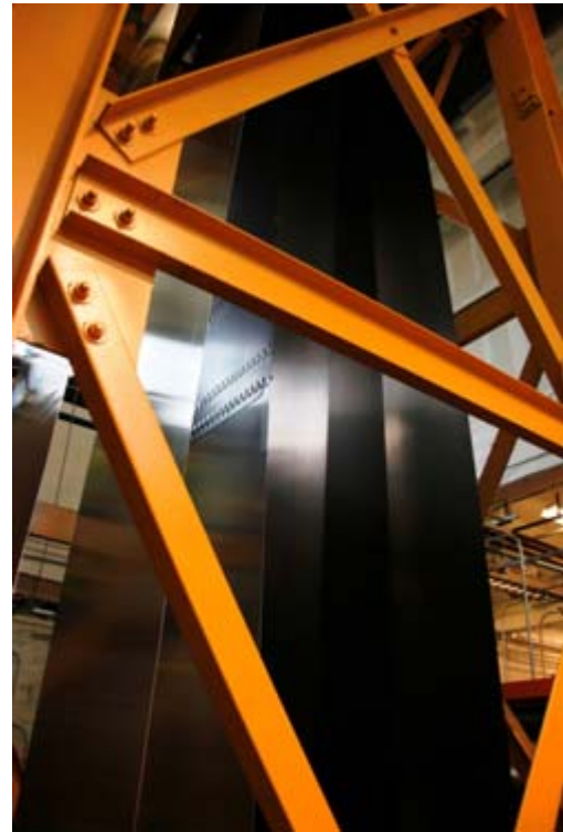
The entry accumulator where the coil is fed to the coating process.
