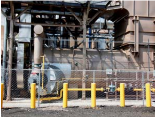
The burner chamber where the system burns off VOCs and recaptures heat for use in the coating process.
