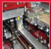
EXIT DRIVE STATION
